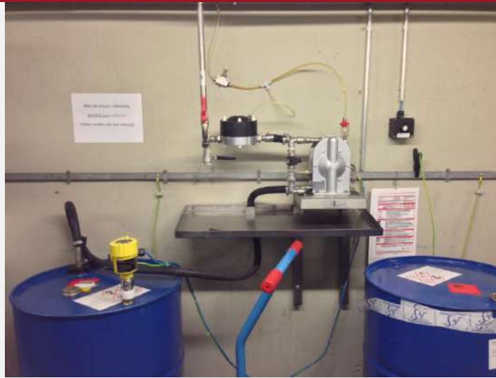
Xylol pump system, 200 liters steel barrels with sensor level
