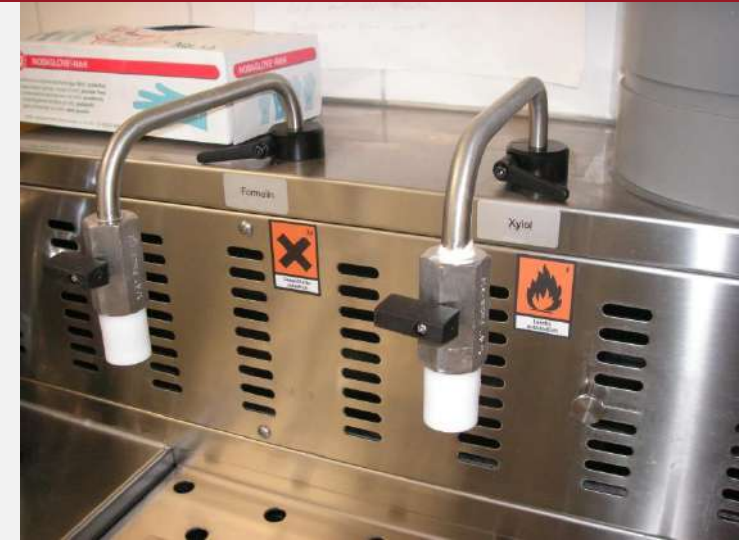
Faucets for formalin, xylol and ethanol
