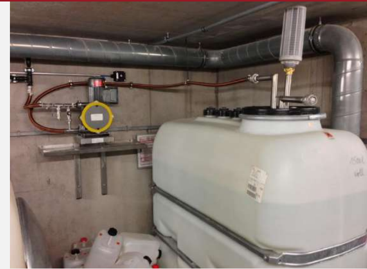
Formalin pump system with supply tank
