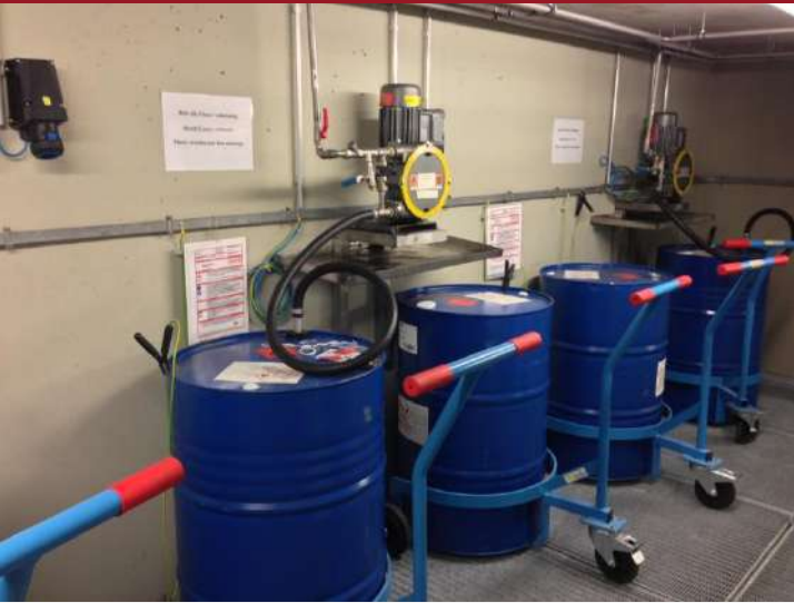
Ethanol pump system (100% ethanol, 96% 1,500 liters ethanol). Stored in 200 liters steel barrels stored in ex protection area
